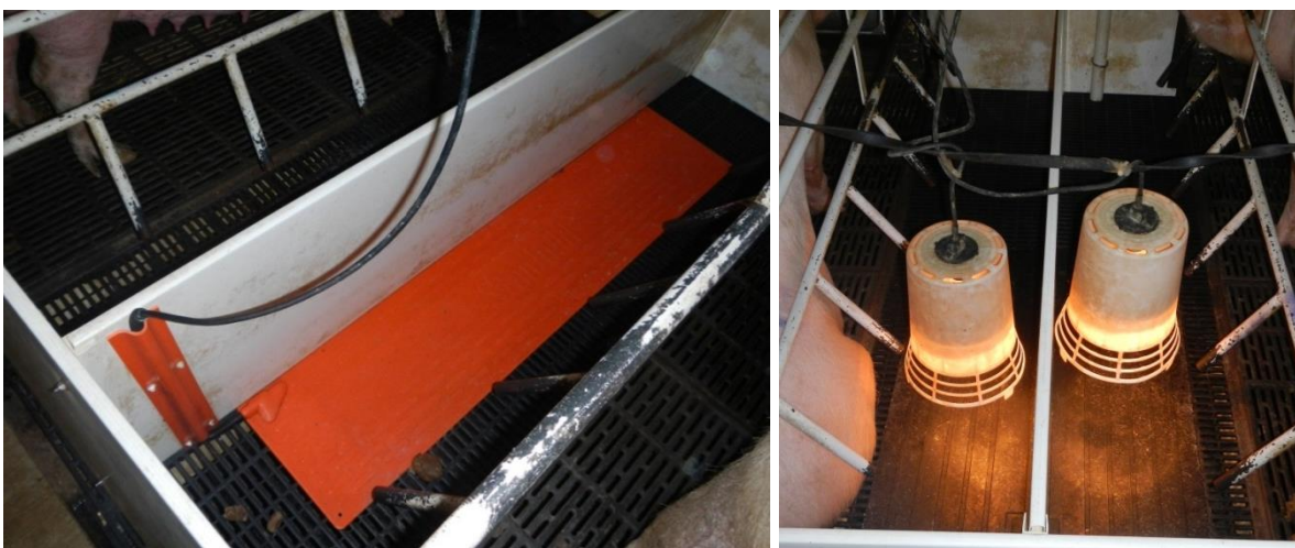
Figure 2. Installed localized heating sources in this study: Stanfield double heat mat (0.6 m × 1.5 m) 290W (145 W each side) heat mat (left) and 125 W heat lamps over a 0.6 m × 1.2 m rubber mat (right).
